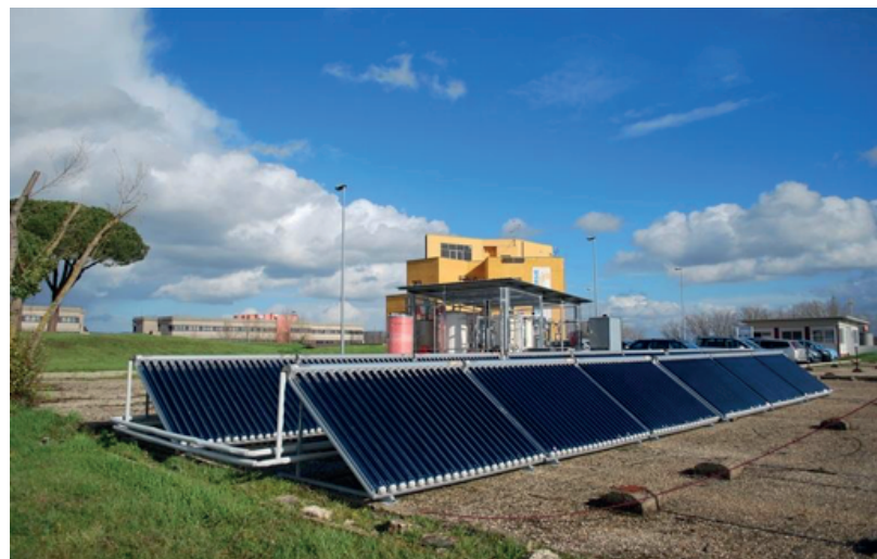
Solar camp with evacuated pipes utilized for heating - cooling
