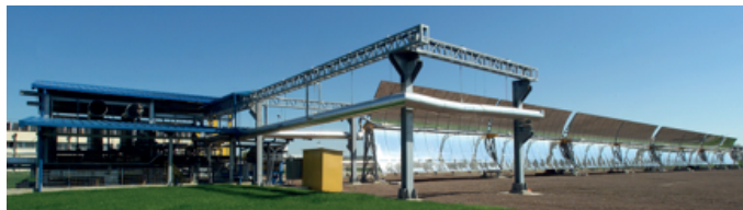
PCS experimental facility
