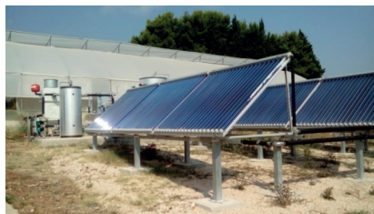
ADRIACOLD Project (solar cooling)
