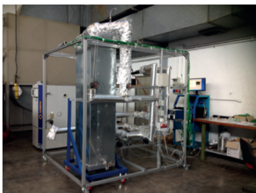
ATES facility (PCM)
