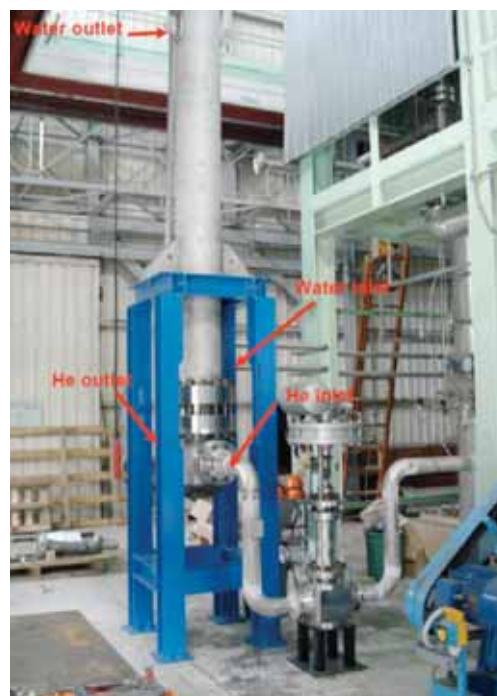
Fig. 3.6 – Helium/water heat exchanger installation
