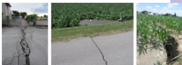
Fig. 19 - Surface effects in San Carlo area (Sant'Agostino Municipality, Ferrara Province).
