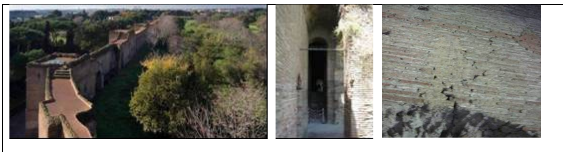
Fig.91. View of the section of the Aurelian Walls subject to monitoring (left); view of one of the monitored tendon in the trench (middle); one of the monitored crack in the wall of a tower (right).
