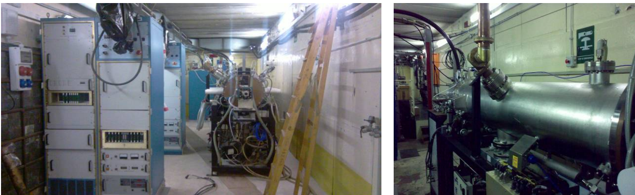
Figure 118 - Pictures of the interior of the proton accelerator bunker: RF power supplies (left), wave guide of the RFQ and the RFQ module up to 3 MeV of proton beam energy (right).
