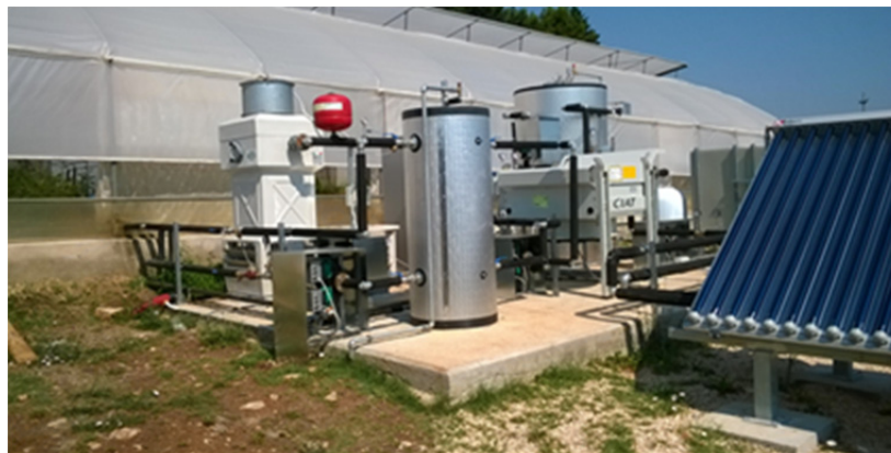
Figure 2. The experimental solar cooling plant.
