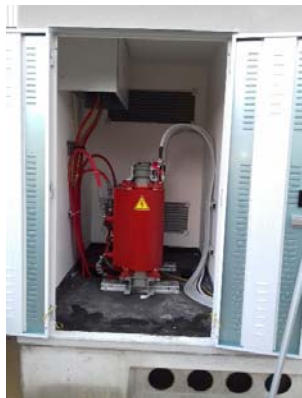
Figure 5. MV/LV substation with a single 400 kVA transformer.
