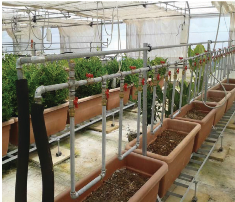
Figure 3. The cooling pipes inside the greenhouse.
