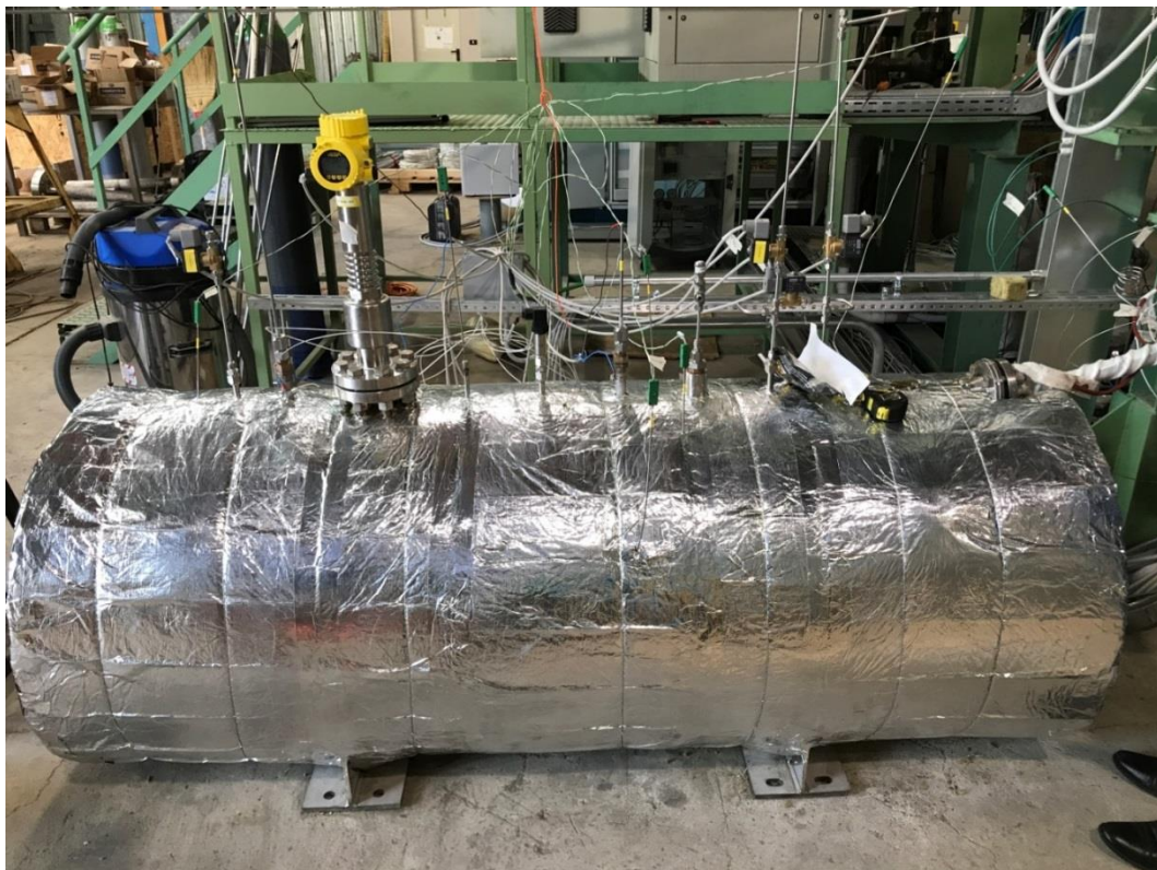
Fig. 8 – S4A storage tank.
