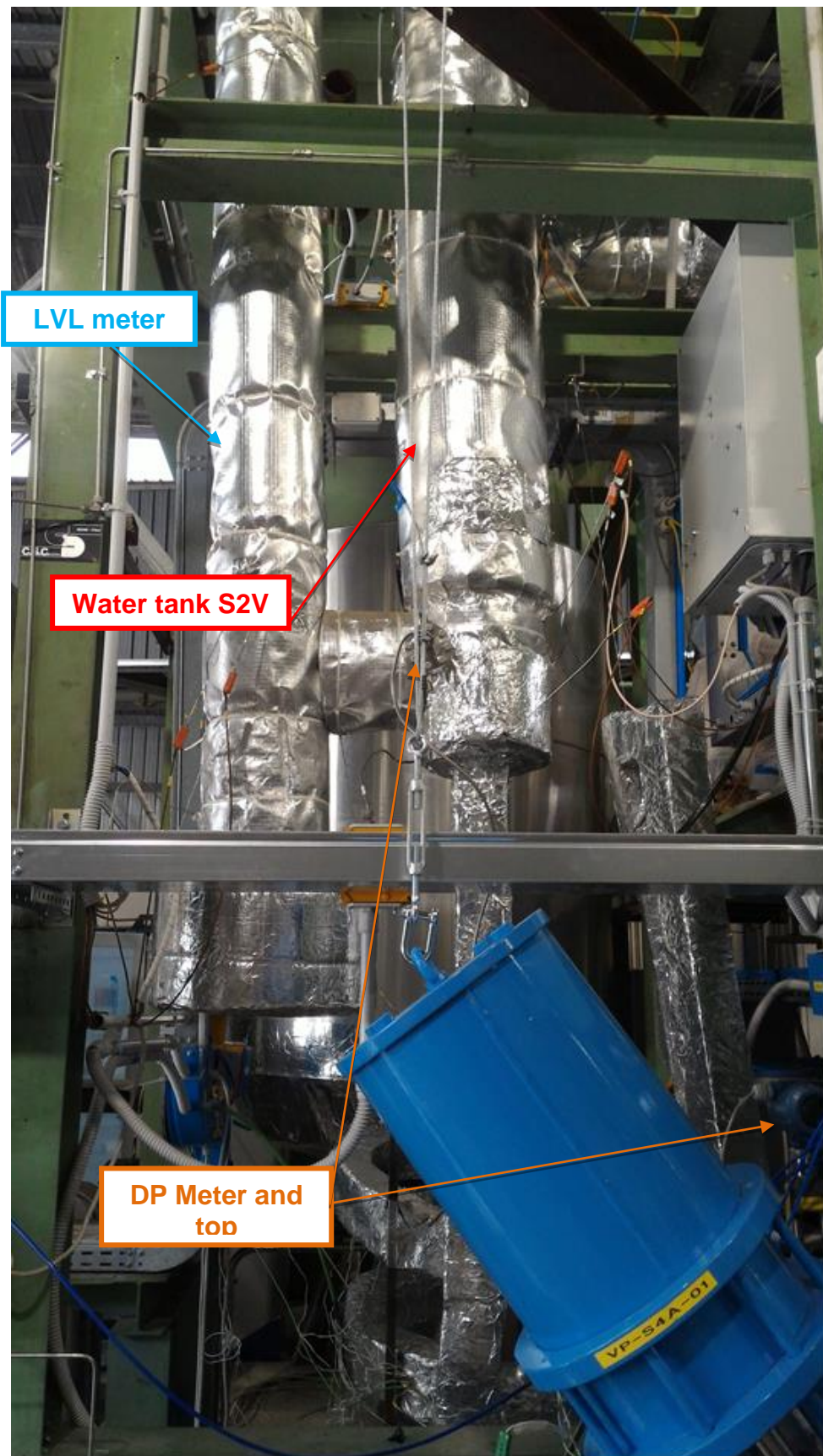
Fig. 5 – S2V and level measurement systems.
