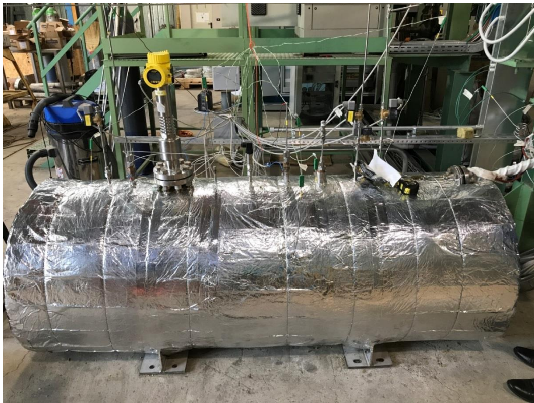
Fig. 8 – S4A storage tank.
