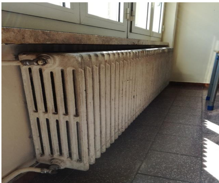
Fig.3.6.2 - Termosifone in ghisa
