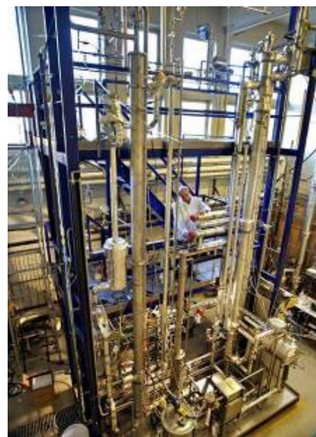
Lab scale absorption pilot plant
