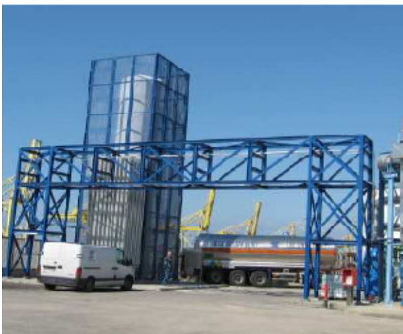
Figure 5 Refill of the oxygen storage tank
