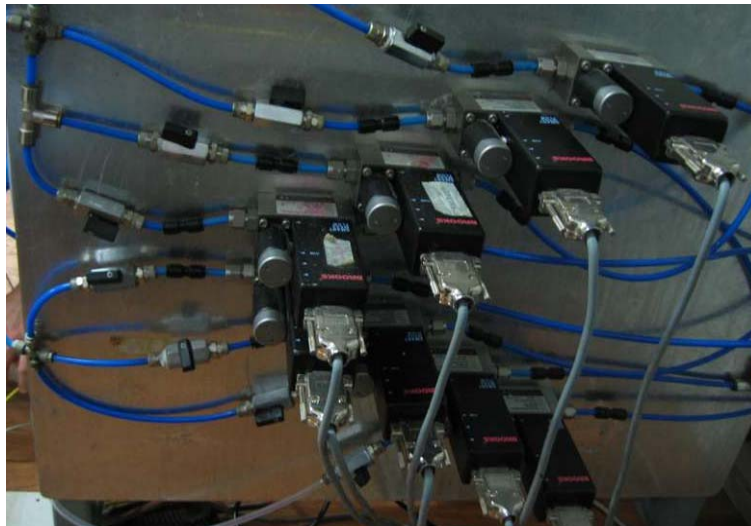
Figura 6. Flow Meter Controllers.
