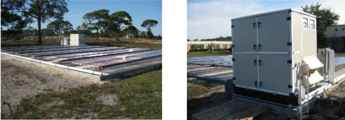
Figure 5.30. AIL Research system installed in Panama City, USA.
