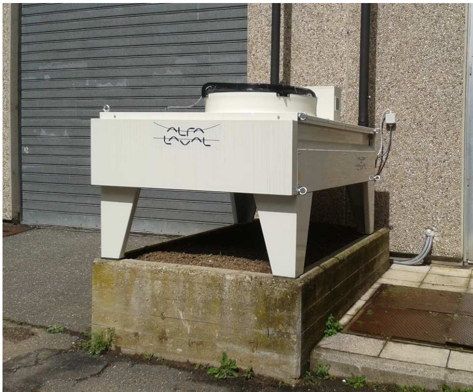
Figura 10. Dry Cooler Alfa Laval
