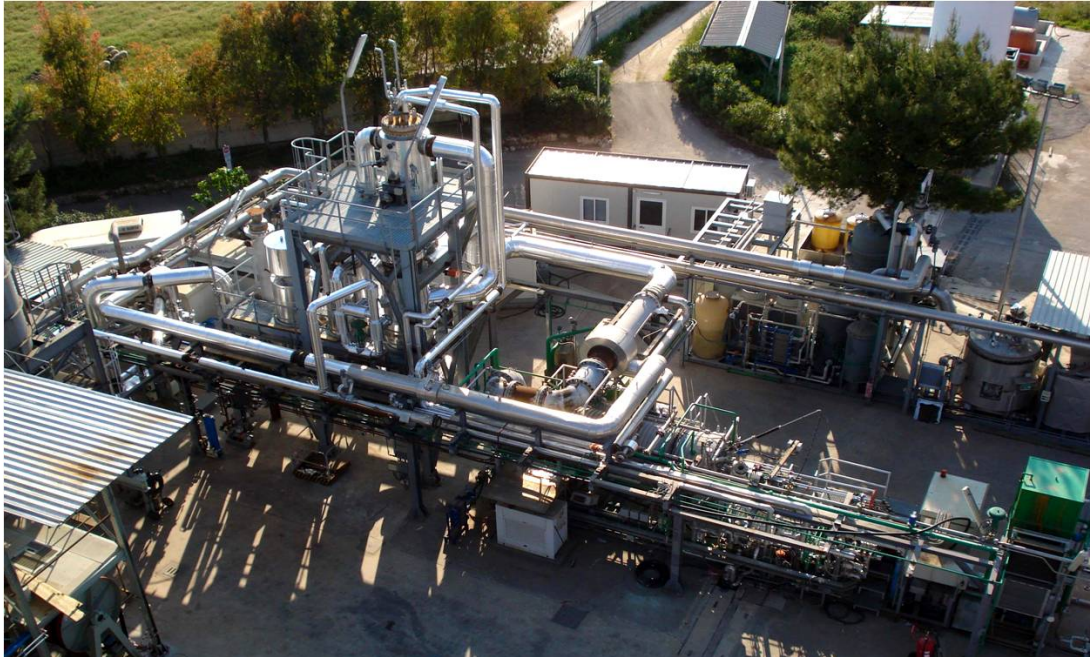
Build-up, in Sulcis area, of a 50 MW th demonstration oxycombustion unit working ant 10 bar pressure
