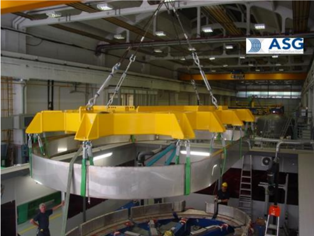
Fig. 11 – WP01 is transferred to cleaning station after VPI
