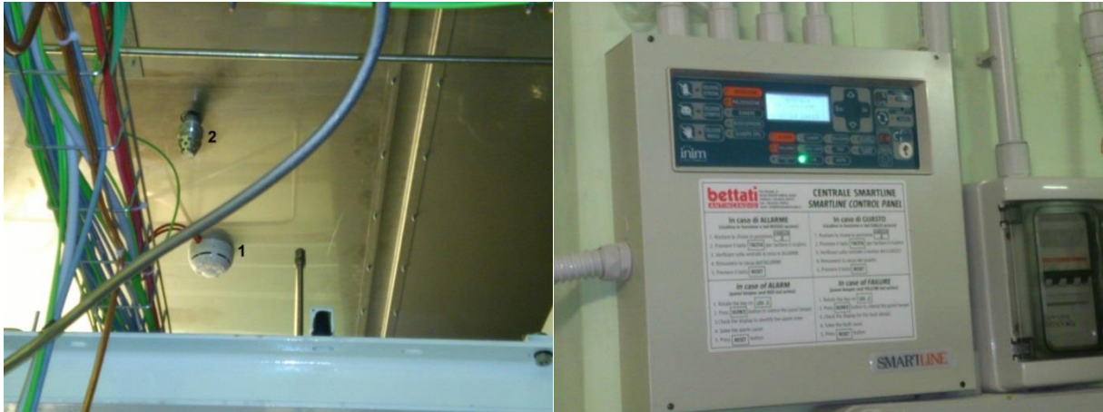
Figure 11: left: inner view of part of the top of the containment box (1: one of the four smoke detectors; 2: one of the two Argon injectors); right: dedicated control panel of the fire extinguishing system
