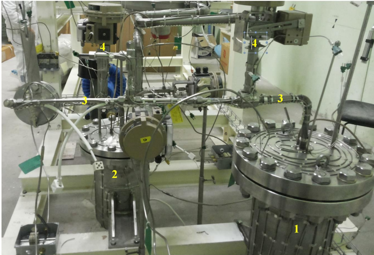
Figure 3: final installation of the Hot Trap inside Lifus 6. 1: Hot Trap; 2: Storage Tank; 3: Pipe connecting the Hot Trap and the Storage Tank; 4: Pneumatic valves
