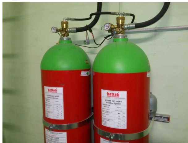
Figure 12: Dedicated high pressure Argon cylinders for the fast injection in the safety box
