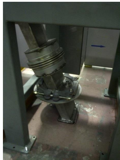
Fig. 23 The bellow on the outlet channel
