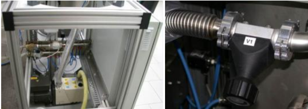
Figure 4: Vacuum pump pipe connections
