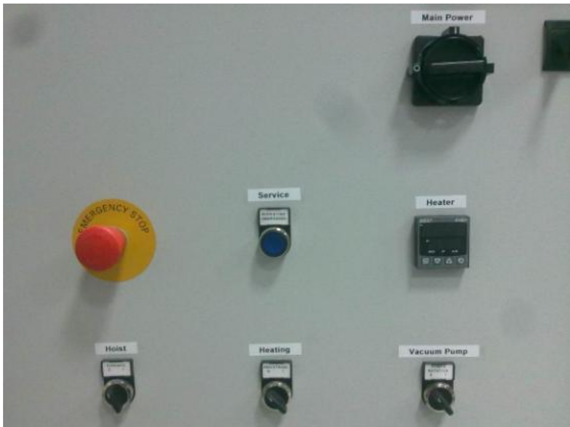
Figure 11: Electrical main panel
