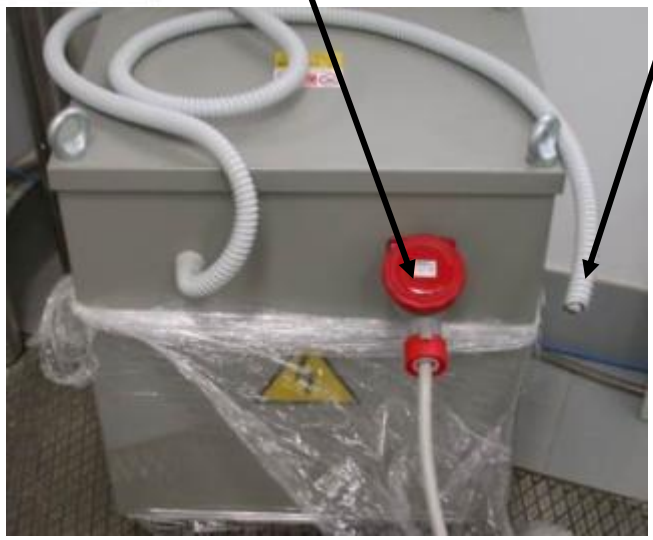
Figure 9: Electrical connections on the transformer TR1
