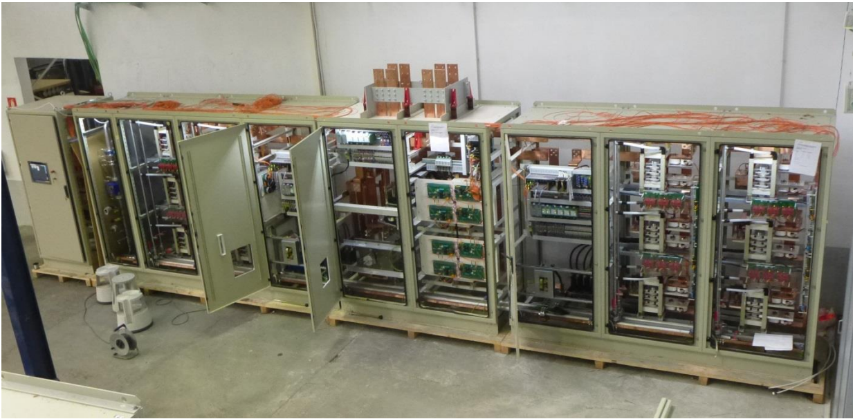
Figure 2 - The view of a FPPCC PS in Jema Laboratories.
