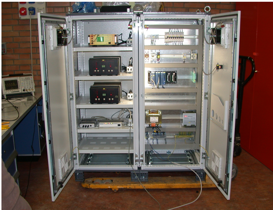
Figure 14: electrical cabinet for the cavitation detector and the resistivity meter
