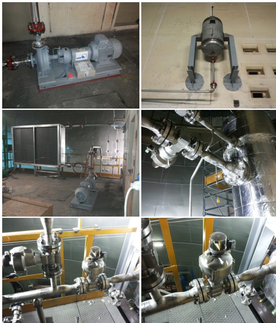
Figure.6: Components of the secondary side of the NACIE-UP facility.
