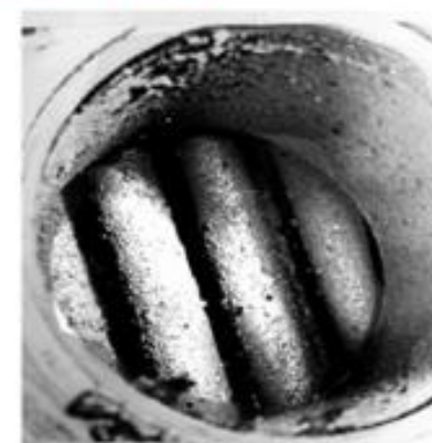
Slag deposit in heat exchanger
