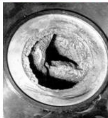
Slag deposit in the circuit during circulation pump tests
