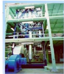
He-FUS3 Facility @ ENEA-Brasimone
