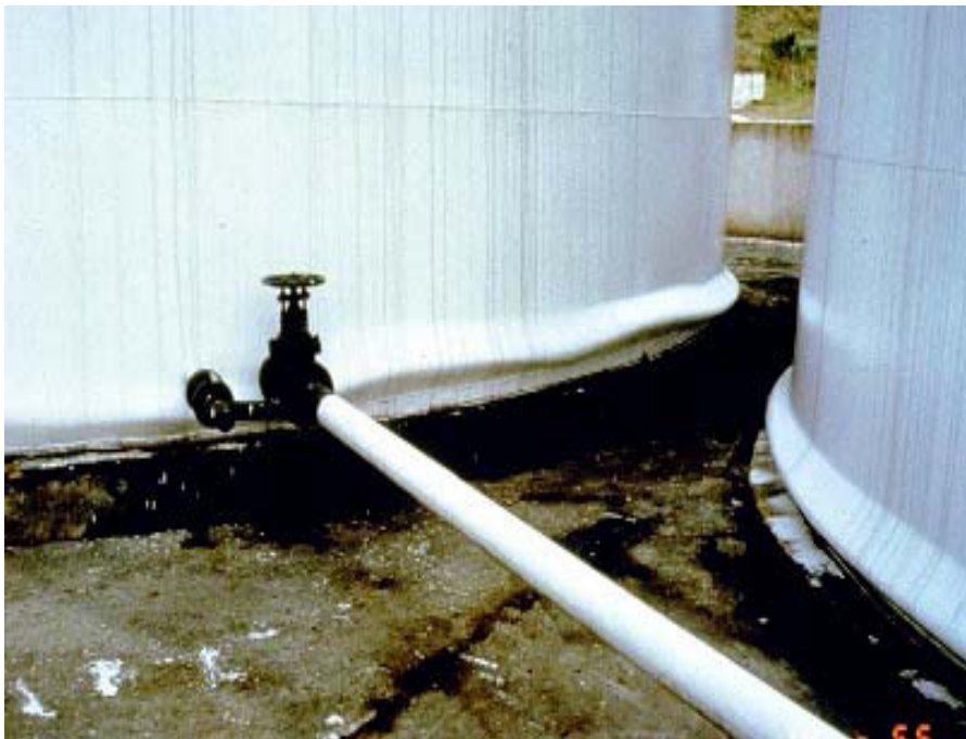
Figure 2 - Elephant's foot buckling deformation
