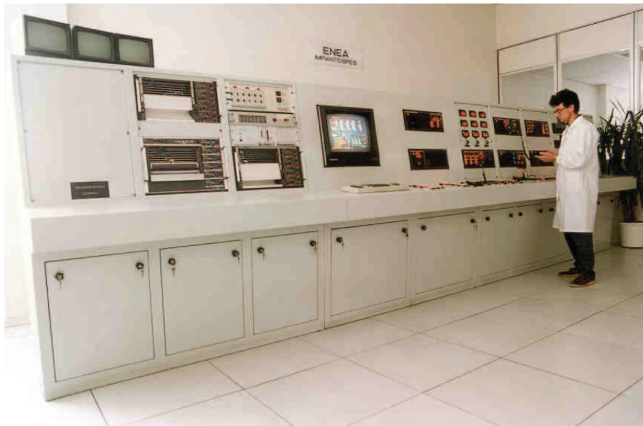
Figure 6 – Test Facility control room
