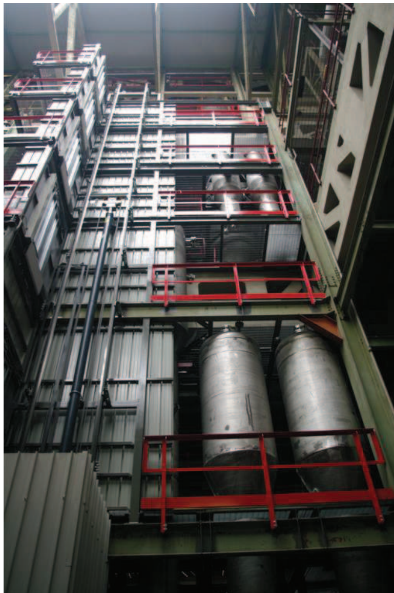
Figure 7 – SPES 3 steel structure
